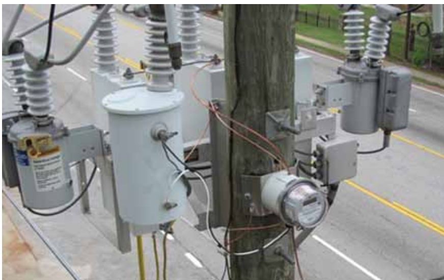
An AMI-based capacitor monitor installed on a switched capacitor bank.
